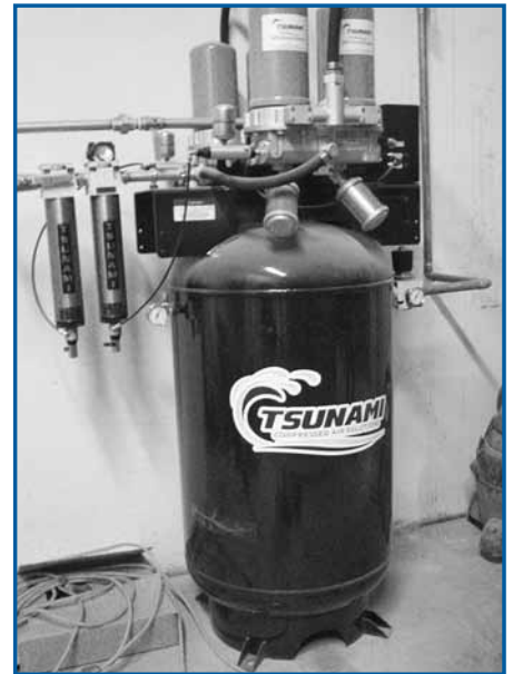
DAA Northwest Auto Body Center invested in a Tsunami—a filtering & drying system for compressed air.
