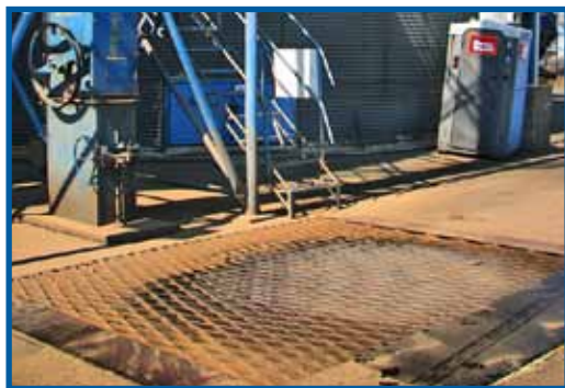
Pictured on the left is a receiving pit with a platform grate over the new baffle system. Product is transferred via conveyor belt to the storage silos.
