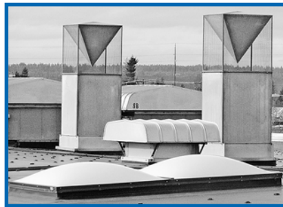
Vertical exhaust stack at least 6' above penetration point of roof with approved stack caps.
